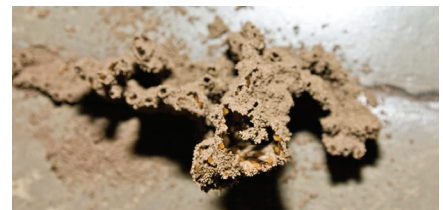
(5D) Swarm tubes emerging from floor crack.
